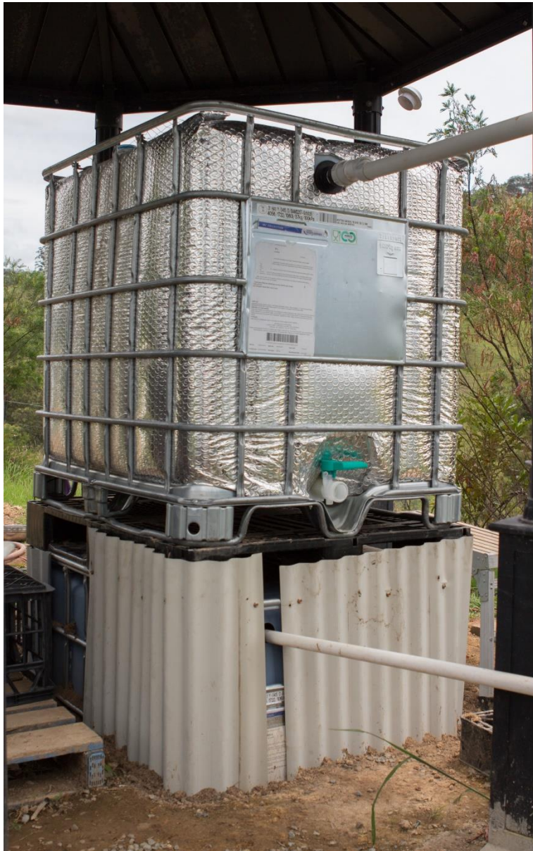
Figure 14 The new fish tank on the top, and the sump tank has been buried in the ground.
