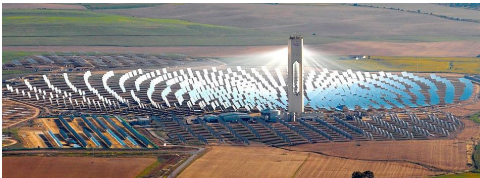
Figure 2.4. Solar power plant (The beauty of solar power plants 2013).
