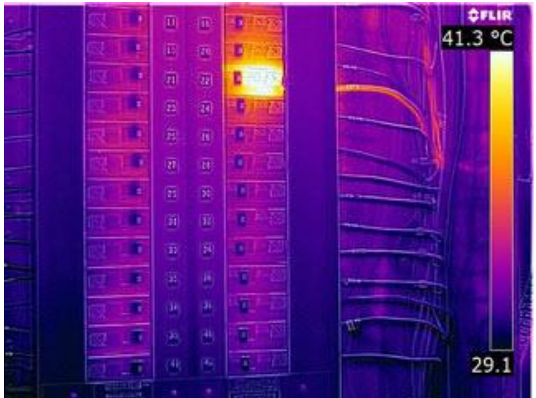
FIGURE 13. Example of thermal diagram showing problem with wire (overheating). (Lumen Electronics, 2016)
