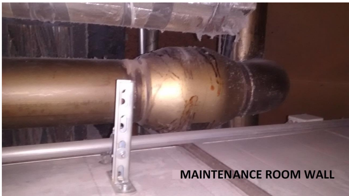
Picture 24. Major pipeline connection and valve in CB 11 spinner floor
