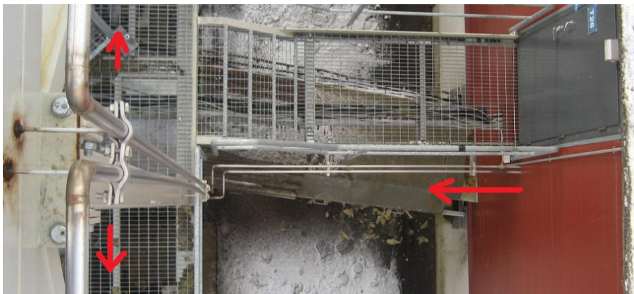
Picture 28. Dust filter unit pipes
