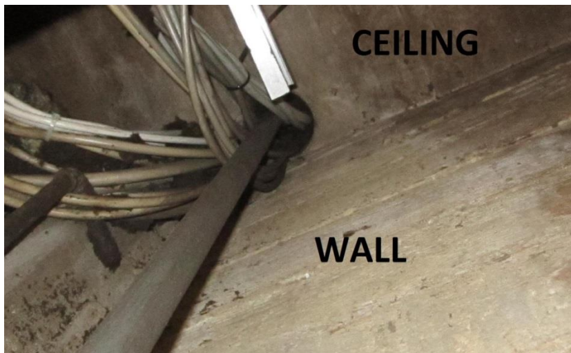
Picture 26. Pipe and cables through the same hole
