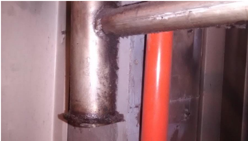
Picture 30. Leaking pipe end cap
