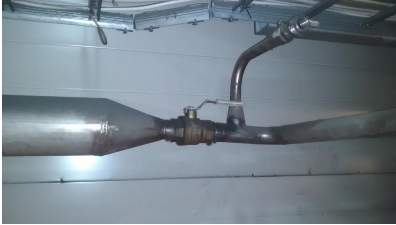
Picture 29. Unconventional reducer in major pipeline in PAL 11 packing
