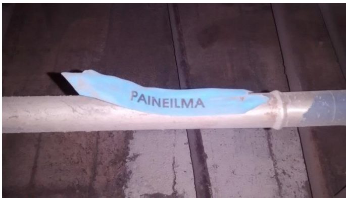
Picture 33. Marked pipe with loose tape
