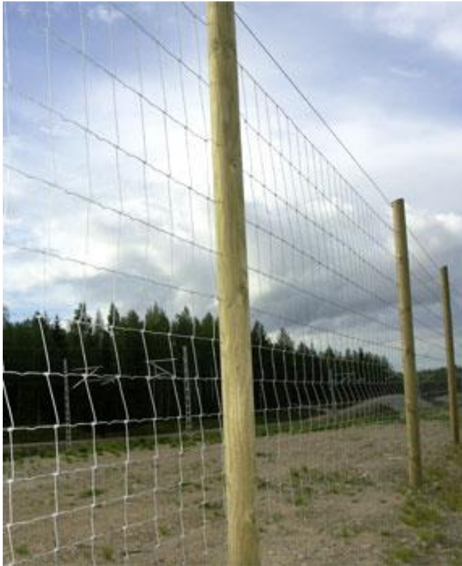
Picture 9. Deer and elk fence (wildlife fence) of VS Turva-Aidat Oy (VS Turva-Aidat Oy 2016).
