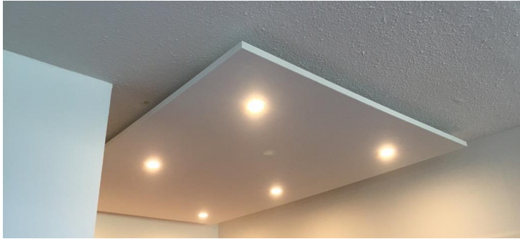
Figure 15. An acoustic ceiling panel with noise sensor controlled lights (Audico 2016).
