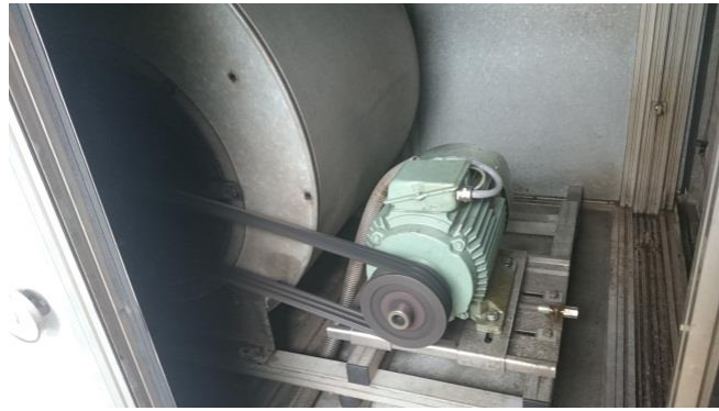
Figure 5 AC motor with a pulley system at Engel
