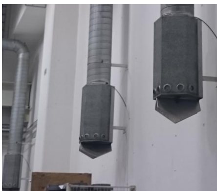
Figure 3 Existing air diffuser
