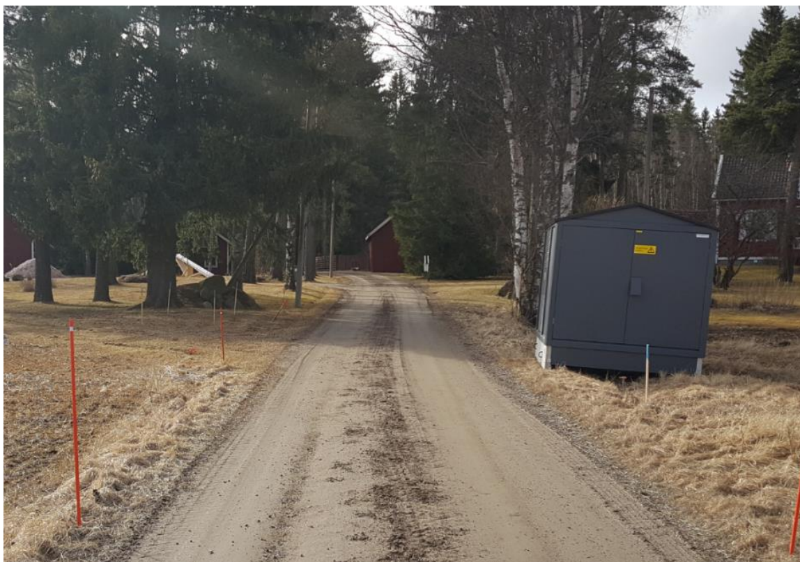
Figur 5, KL-INDUSTRI Elit 4 marktransformator
