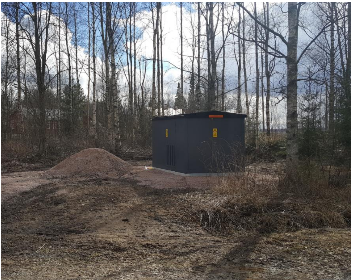
Figur 4, ABB Mercury 12CC marktransformator
