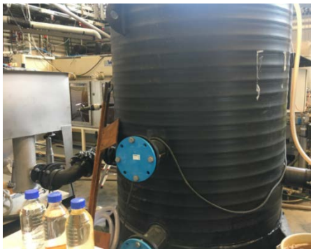
Figure 19. New flocculation tank inside
