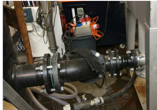
Figure 18. Big in take pipe
