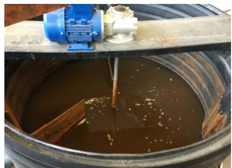
Figure 20 New flocculation tank
