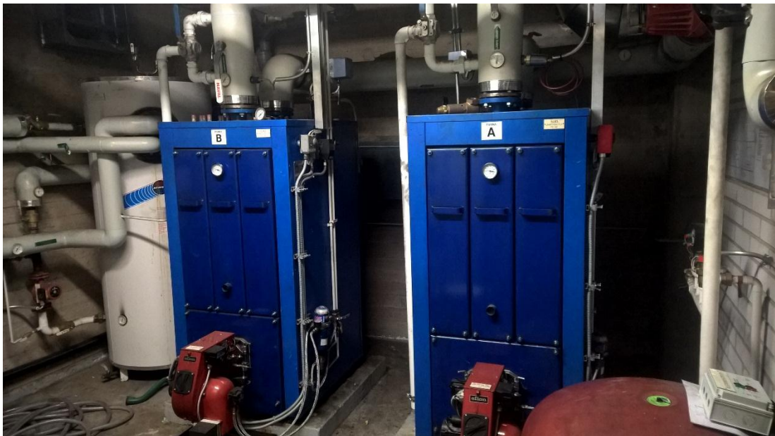
Figure 2 The two oil boilers in the technical room (Author, 2016)
