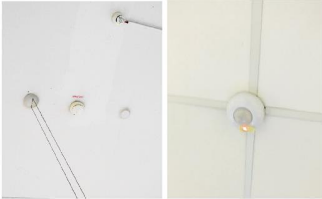
Figure 11: Barely noticeable smoke alarms on the ceilings of University of Tuebingen (left) and Poznan University of Economics (right).
