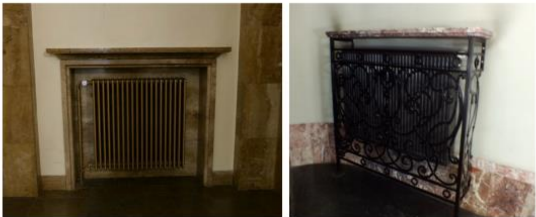
Figure 22: Brass radiators with matching marble frames in University of Tuebingen (left) and with decorative metal frames in Adam Mickiewicz University (right).
