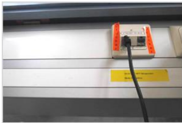
Figure 8: Cables are covered by matching-colored panels (taken in University of Tübingen)
