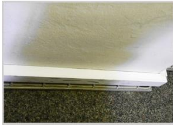
Figure 7: Cables at the foot of a wall coated in color-matching paint (University of Mannheim)
