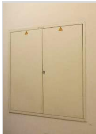
Figure 6: Doors to electricity system control with small, yet visible warning stickers (University of Mannheim)
