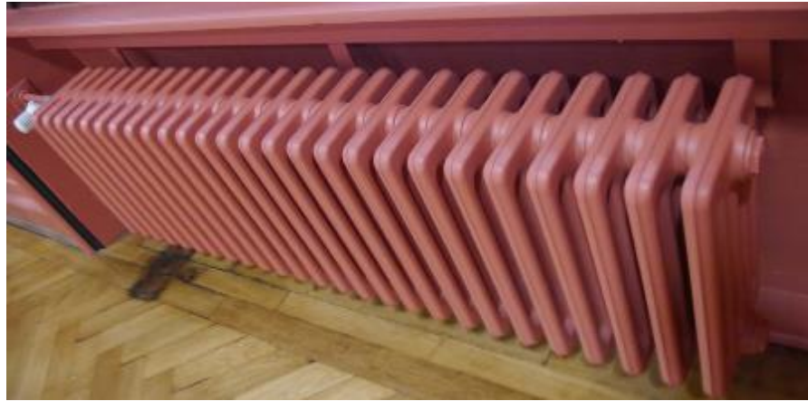
Figure 13: Radiator painted the same colour as the window pane above, as seen in University of Heidelberg.
