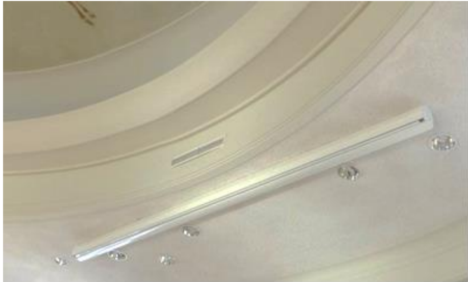
Figure 17: Well-hidden ventilator hatch on the ceiling of conference room (seen in Adam Mickiewicz University)
