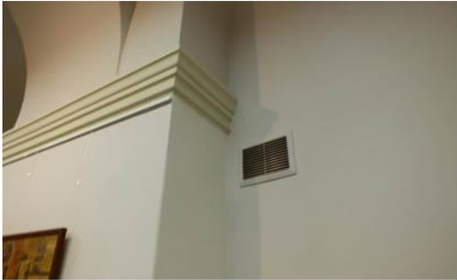
Figure 15: Ventilator hidden next to an intruding wall, as seen in University of Wroclaw.
