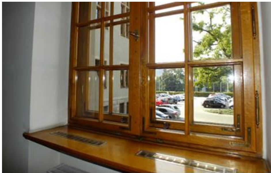
Figure 16: Ventilator hidden inside wooden window pane in Adam Mickiewicz University.
