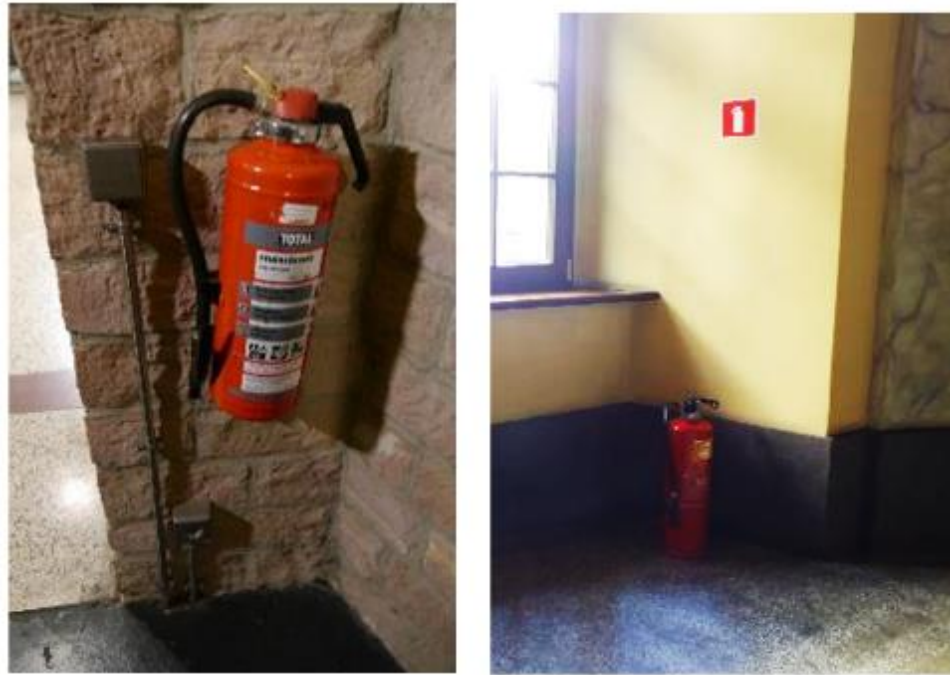
Figure 33: Fire extinguisher put in the corner of the corridor, exclusively from the main part. (Left: University of Heidelberg, right: Adam Mickiewicz University)
