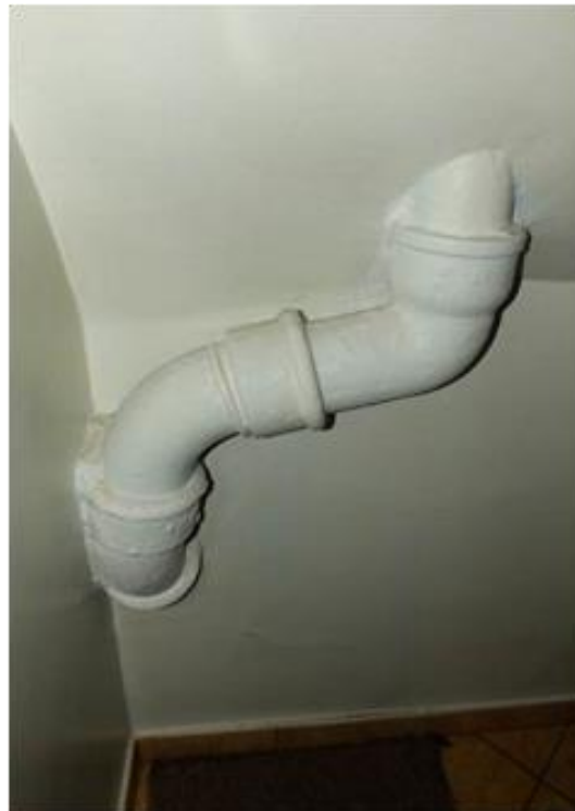
Figure 12: Part of the water system in Poznan University of Economics, well hidden in the basement in a corner.
