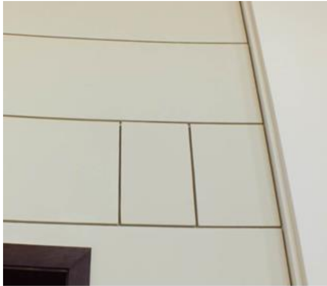
Figure 9: Removable panels to access the electricity system. (Taken in Adam Mickiewicz University)
