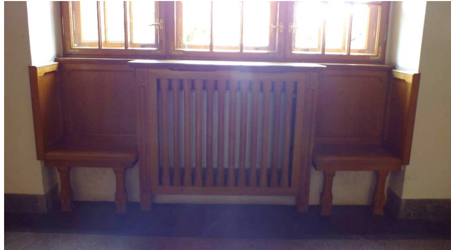
Figure 21: Radiator with a wooden covers and benches at the sides (as seen in Adam Mickiewicz University)
