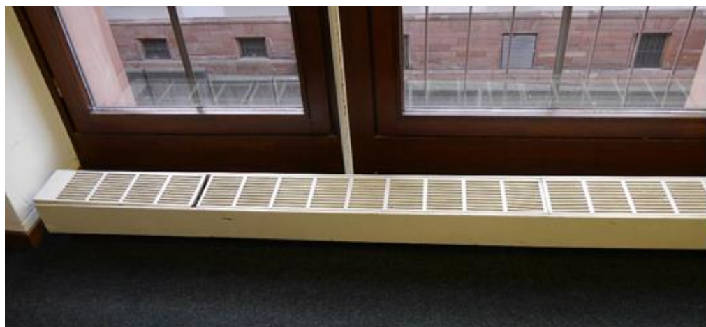
Figure 14: Small ventilator placed along the window pane, as seen in University of Heidelberg.
