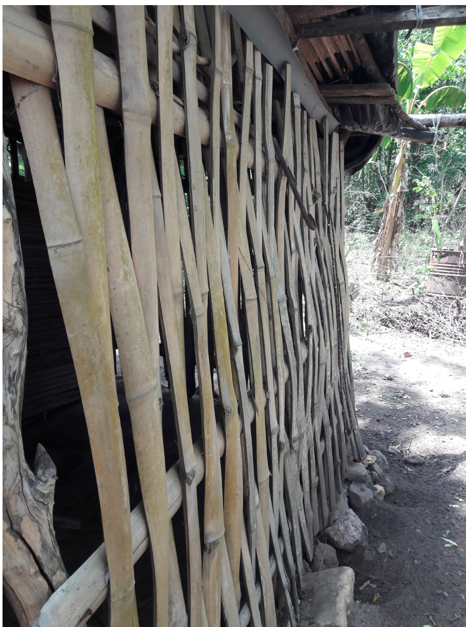
Image 2. Pit toilet constructed with a locally available material bamboo (photo Maarit Virtanen).
