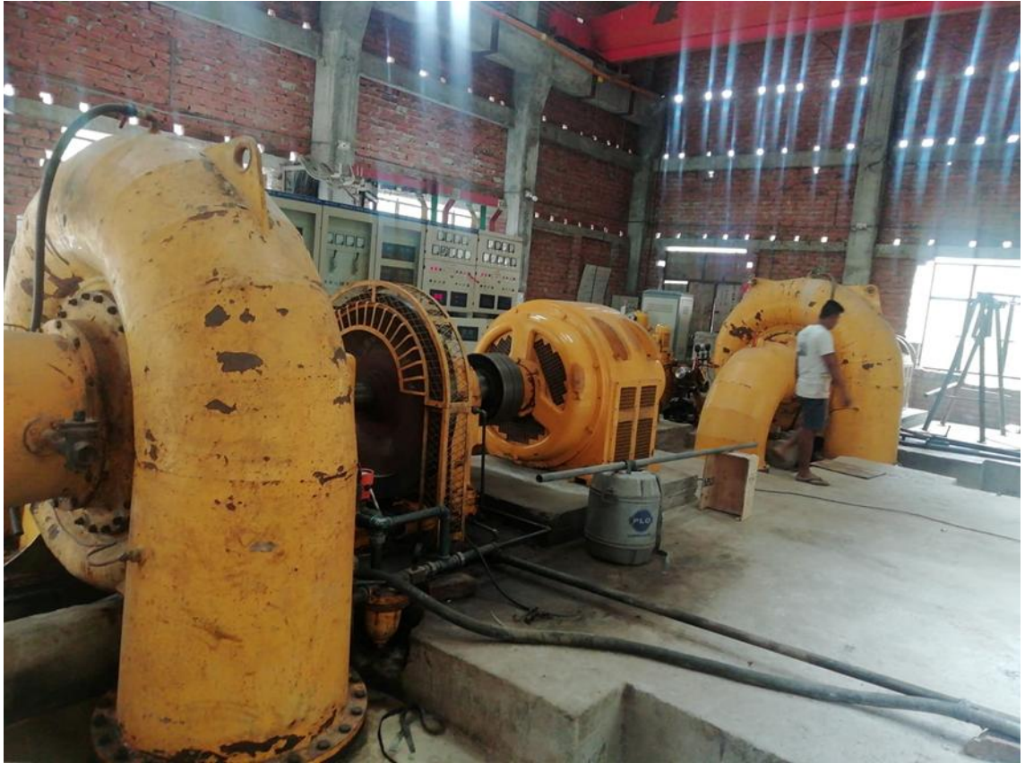
Figure 2. Turbine and generator operating inside the powerhouse.
