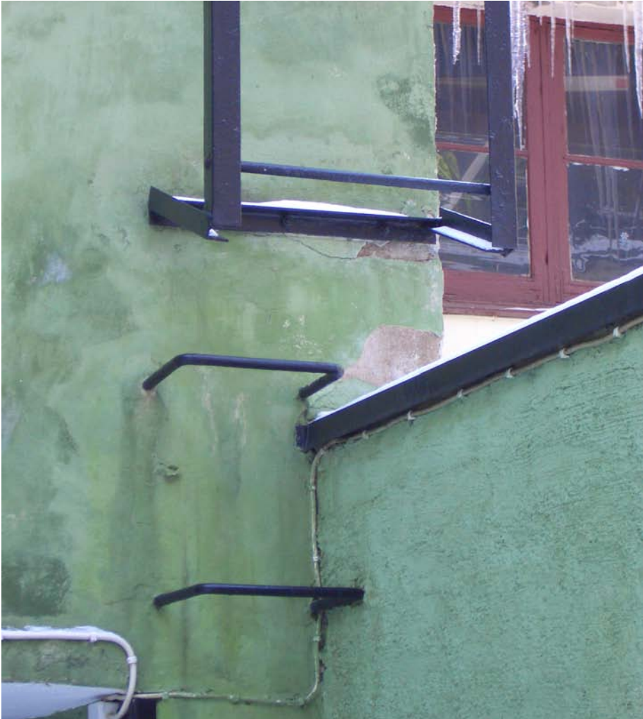
Figure 4. Multiple problems on both rendering and lime wash caused by bad detailing, rain and frost.
