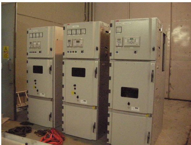
Picture 2, Switchgear cabinets
