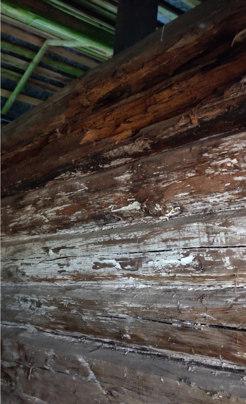
PICTURE 1. Rotten and partly damaged wood caused by humidity.
