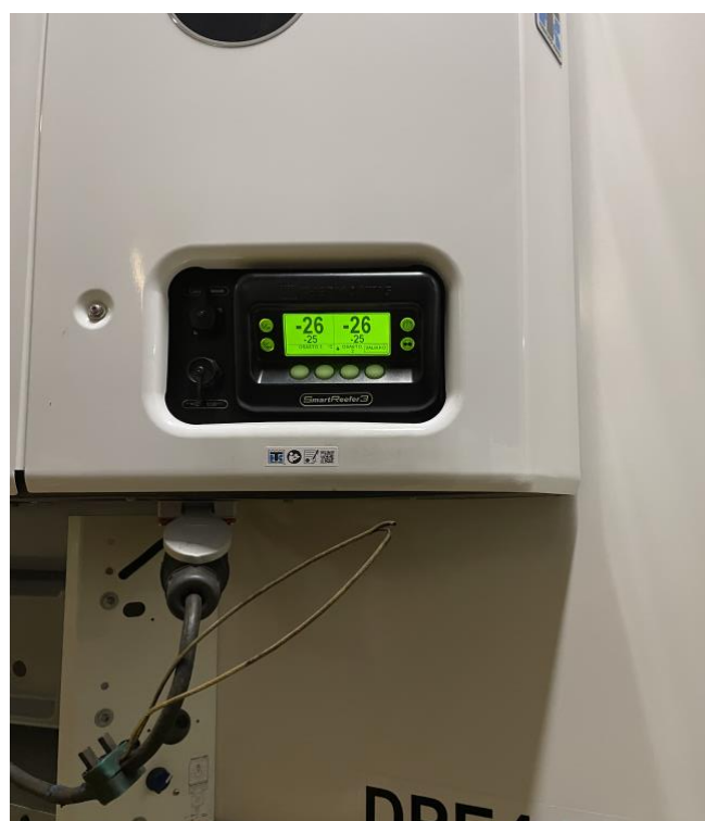
Figure 9: ELE-unit control panel.
