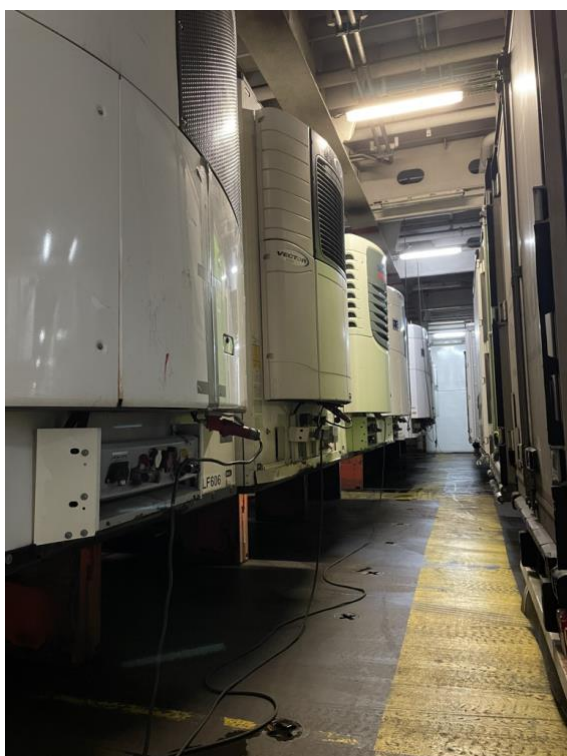
Figure 7: ELE-units connected to ship's electricity.
