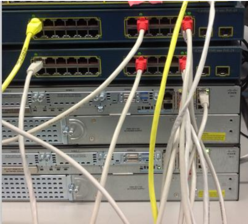
FIGURE 12. setting the ports on the switches to make the virtual interface. ( Photograph by Chen Lu, 2014.)
