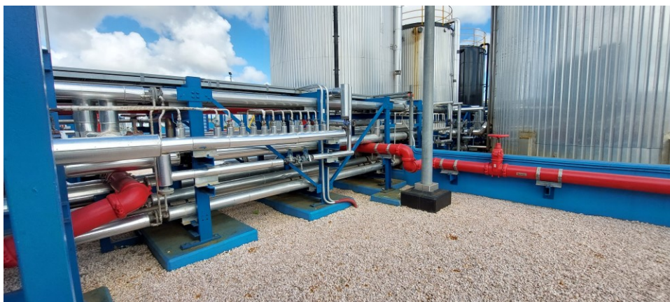
Figure 2. Pipe rack with insulated pipes. (Wärtsilä 2020.)
