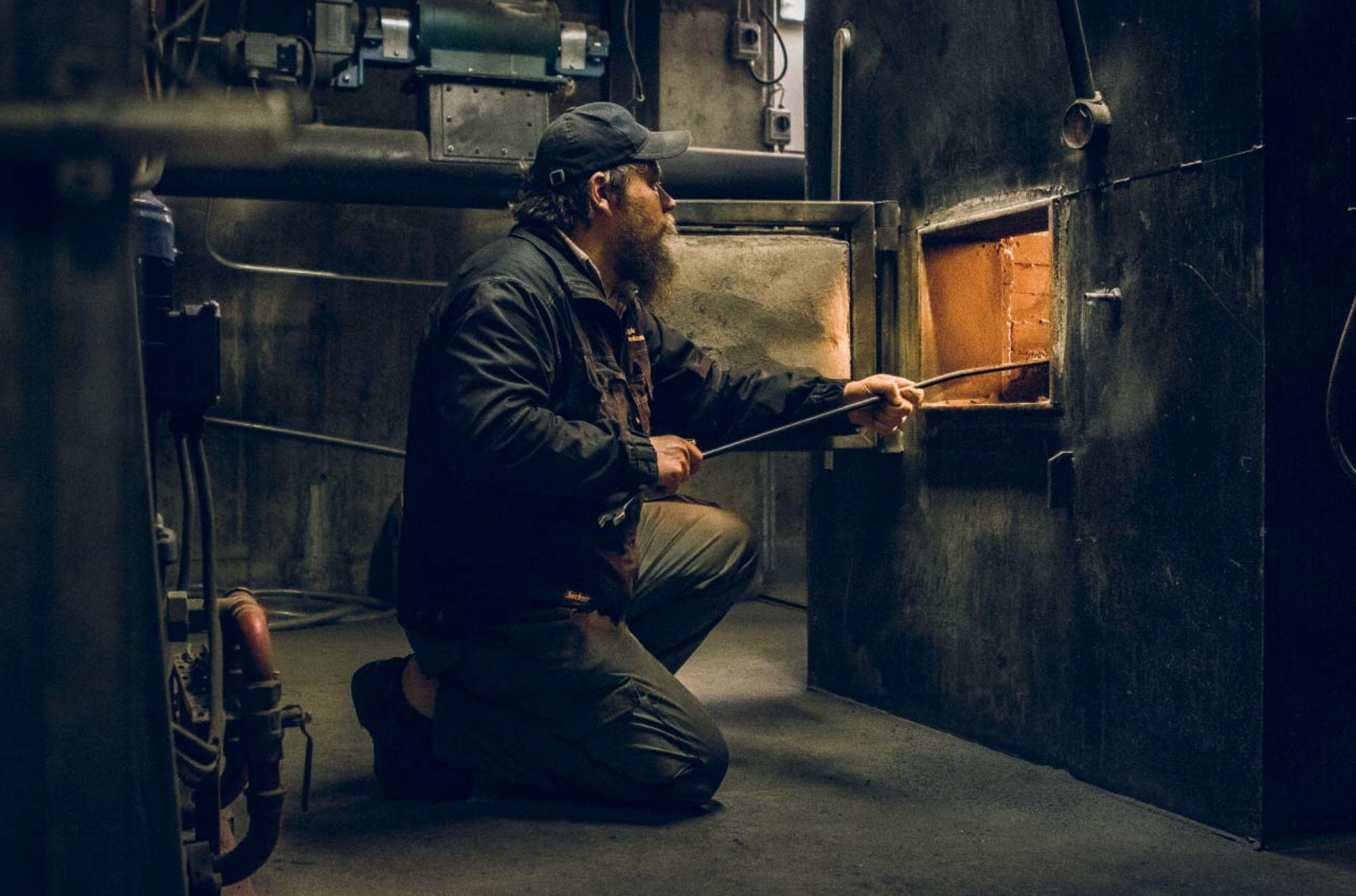
The Eno Heating Cooperative owns three wood chip heating plants, taking care altogether of eight biomass boilers. The cooperative buys the energy wood for chip production from the local forests. Local energy wood markets increases regeneration of the forests and by using wood chips, the community saves 1 million litres of light heating oil annually.
