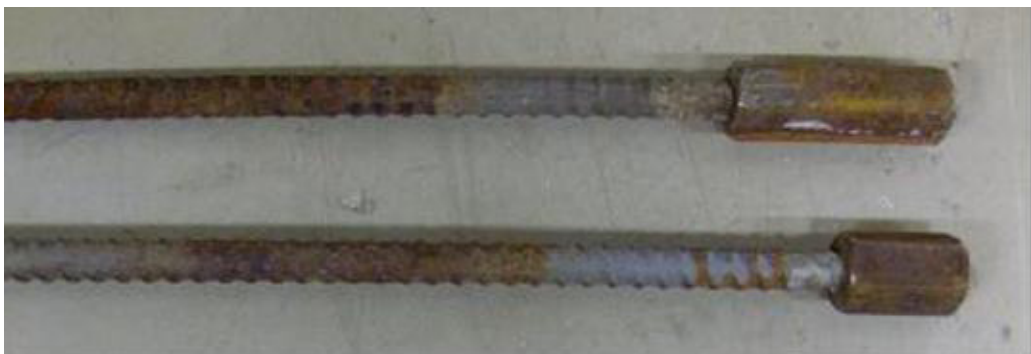
Figure 9 Corrosion on bars used as pre-stressed bars.
