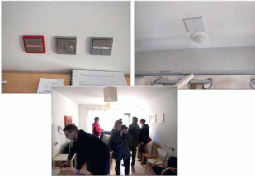
Figure 4. Various technologies installed in the apartments at the Great Northern Haven
