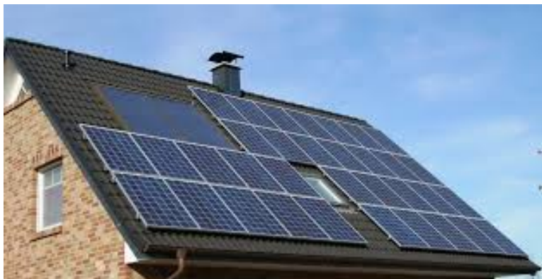
Picture 1. Solar panels
