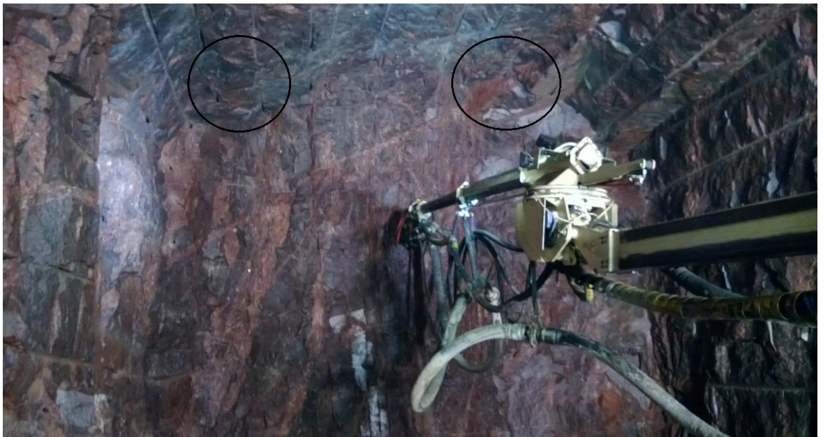
Figure 2. Under breaks at the face due to inaccurate drilling (photo by Olli Weman)
