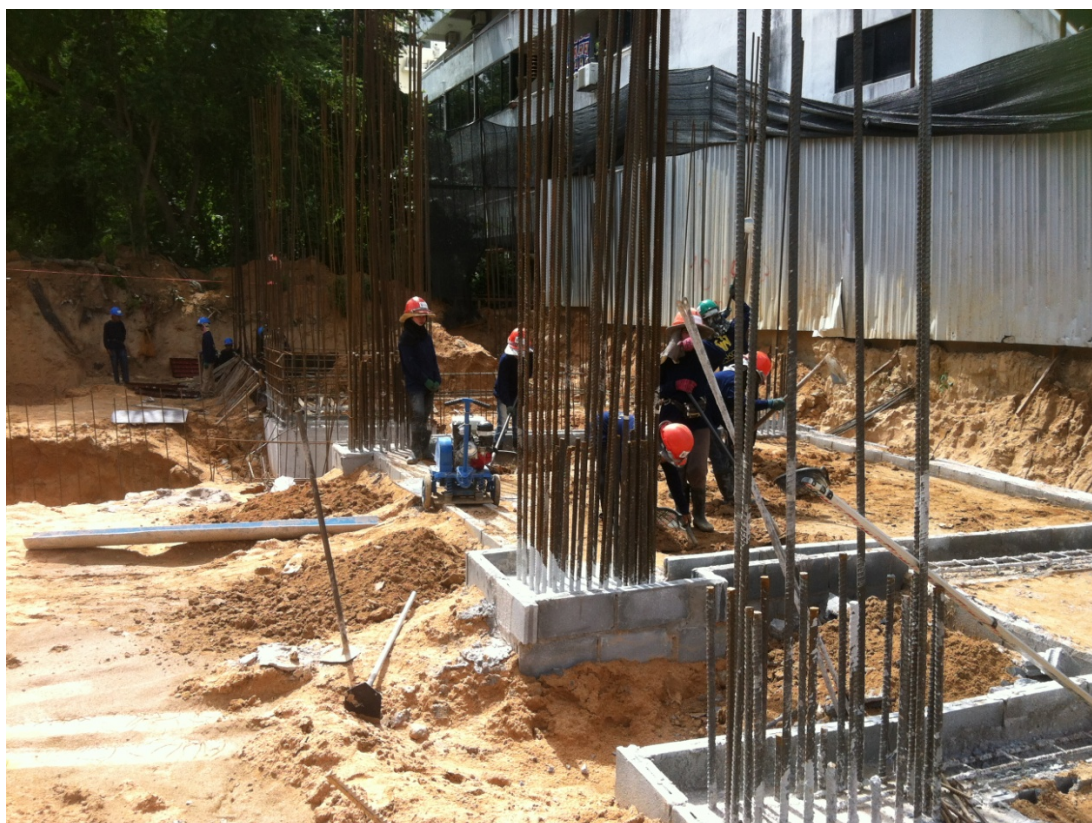
IMAGE 3. Foundation work of cast in place residential building. Picture is taken from Scanditech's project in Pattaya (Kuronen and Turunen 2013-07-24).
