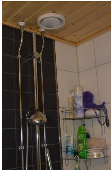
FIGURE 7. Exhaust air diffuser in the bathroom
