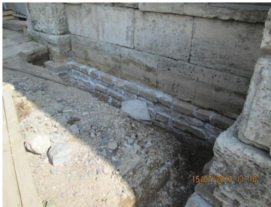
Figure 11.7 Restoration process of rubble foundation masonry. Punching and embedment of the masonry seams
