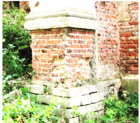
Figure 10.32 Destroyed top of the foundation, destroyed socle, top of the socle
