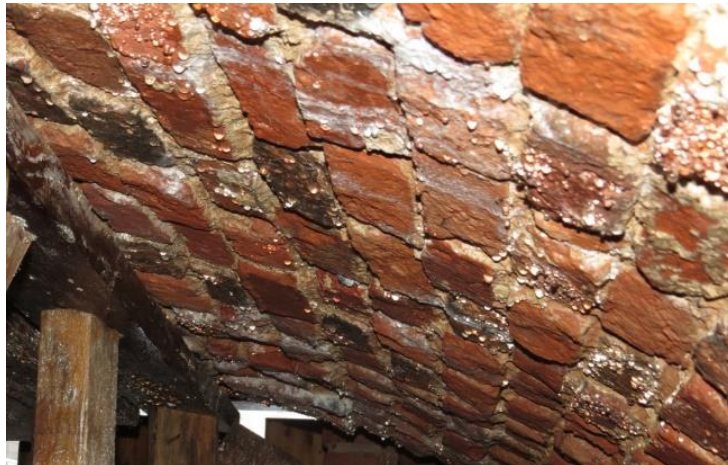
Figure 11.10 Soaking of the brick masonry vault because of waterproofing malfunction of terrace
