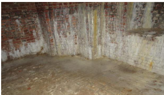
Figure 7.1 Water leakages through brick masonry. Salt sediments on the walls and floor
