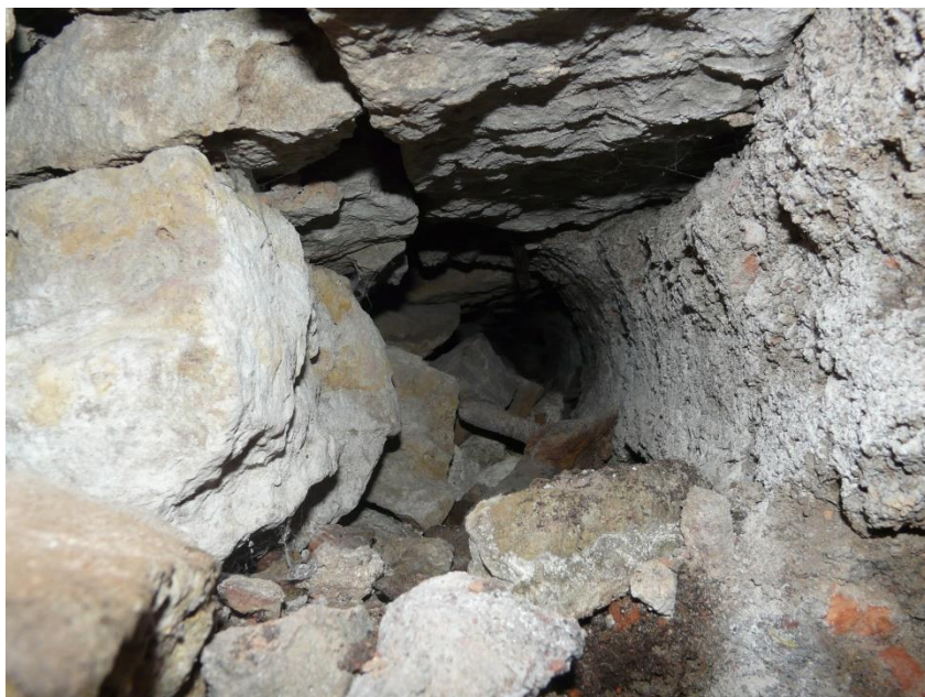
Figure 6.1 Apraksin Yard, house 4, Saint-Petersburg. Totally destroyed wooden logs because of the rot processes
