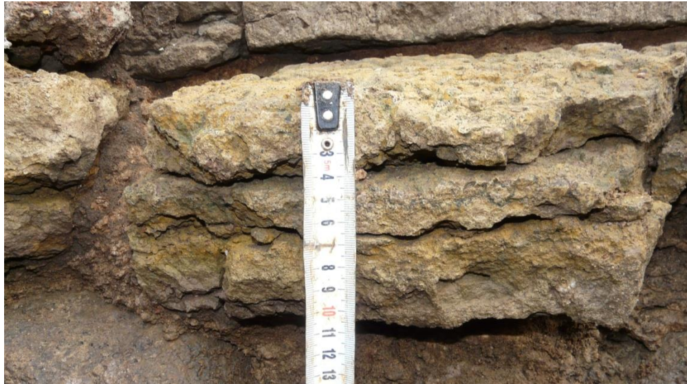
Figure 6.3 Destruction of the foundation masonry made of limestone and lime-sand mortar after prolonged influence of the water and frost
