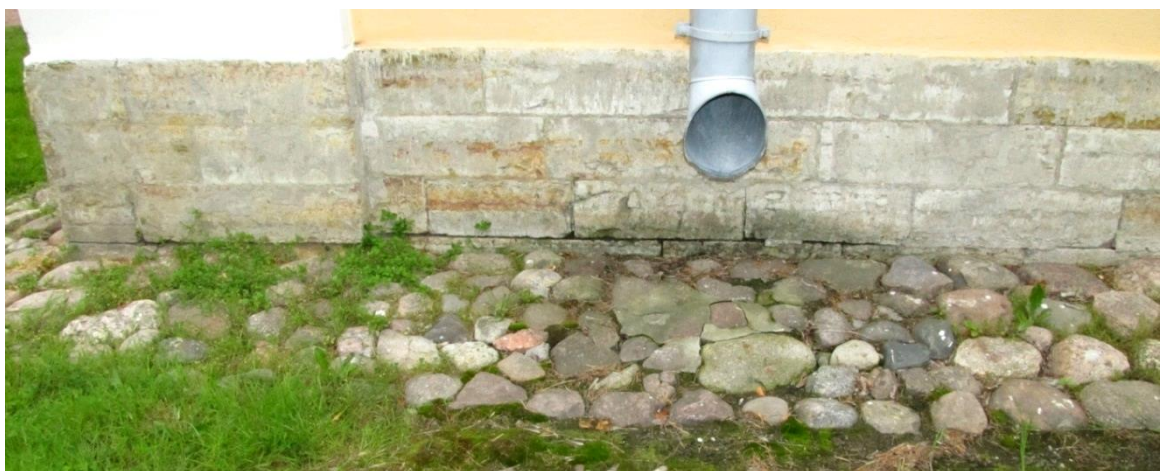
Figure 10.15 Blind area made of small granite stones. Insufficient water removing from the wall. Soaking of the materials and developing of the bio destruction by plants and mold
