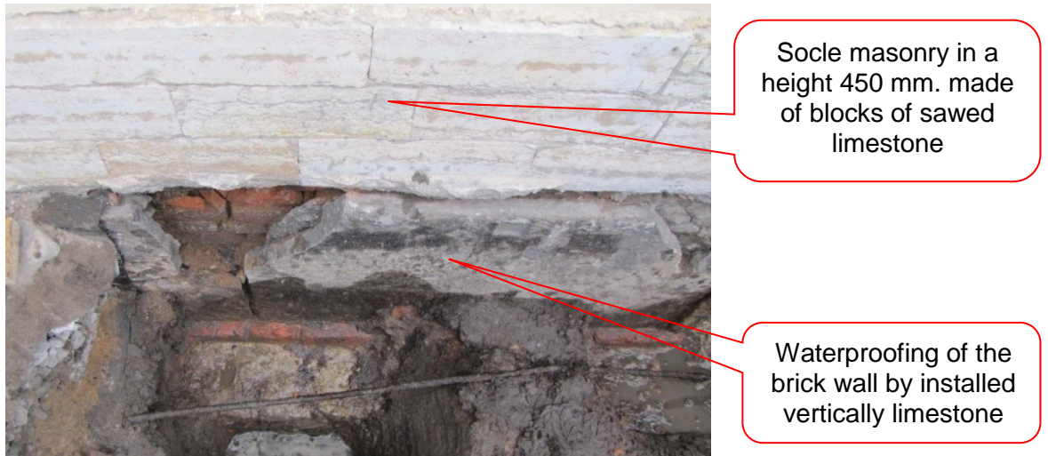
Figure 10.7. The outer vertical foundation waterproofing of the house №6 A, which are made of limestone slabs, and installed vertically to the foundation end
