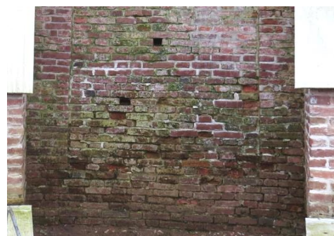
Figure 7.2 Biological destruction of brick masonry as a result of hydro isolation malfunction
