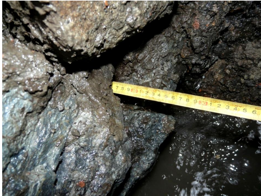
Figure 10.23 Elution of the lime-sand mortar of the foundation masonry to the depth of 1 brick layer as a result of elution during long building exploitation period (>100 years)
