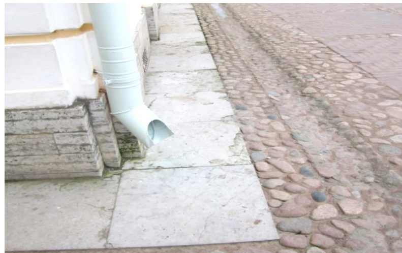
Figure 10.18 Peterhof. Grand Palace. Socle made of sawn limestone to the lime-sand mortar. Blind-area made of limestone. Heated outfall from the roof through the outer drainage gutter
