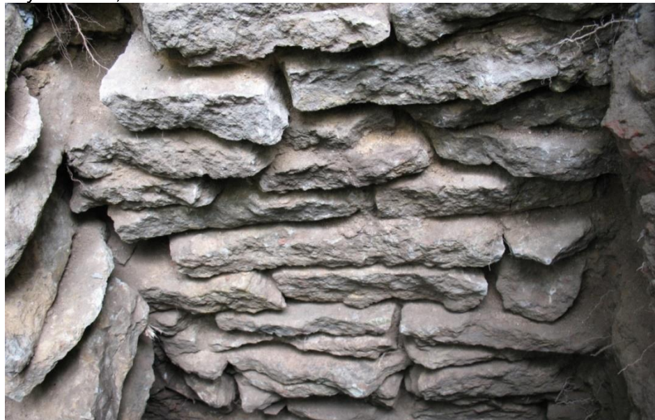
Figure 10.26 Saint-Petersburg. Sadovaya Street house 8/7, 2008 year. Elution of the masonry mortar in the outer layer of the foundation in the period of a long building exploitation (>100 years). Absence of hydro isolation. Absence of vertical foundation waterproofing
