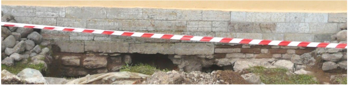
Figure 6.4 Damages of the foundation in the place of the entrance of the engineer networks. Replacement of destroyed limestone in the socle by bricks
