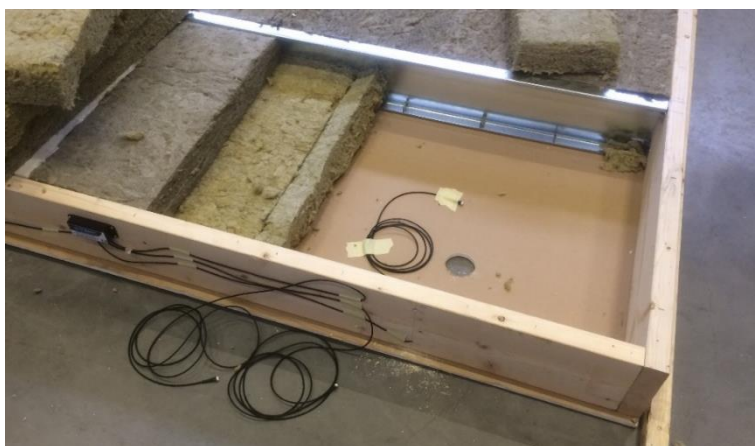
Figure 13. Assembly of Sensors in Zone 1.2
