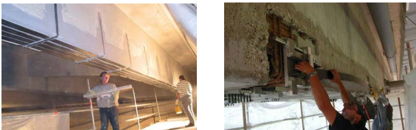
Figure 1. Two examples of the application of CFRP-strips to a bridge construction (HP-TL); left: Retrofitting by adhesively bonded slack CFRP-strips; right: Post-strengthening using a pre-stressing system.
