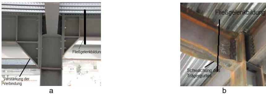
Figure 5. Constructive measures for the development of plastic hinges at the beam end.
