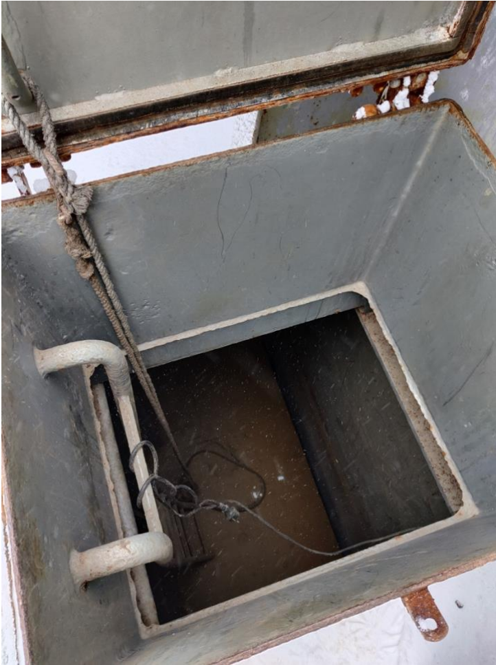
Figure 25 Forward cargo hold entrance. Good to check runoff marks from the sides to detect possible leakage. (Matti Heinonen 2021)
