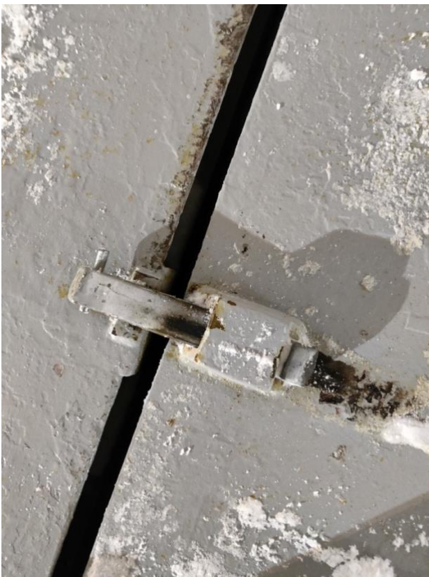
Figure 37 Cross-joint cleat close position. (Matti Heinonen 2021)
