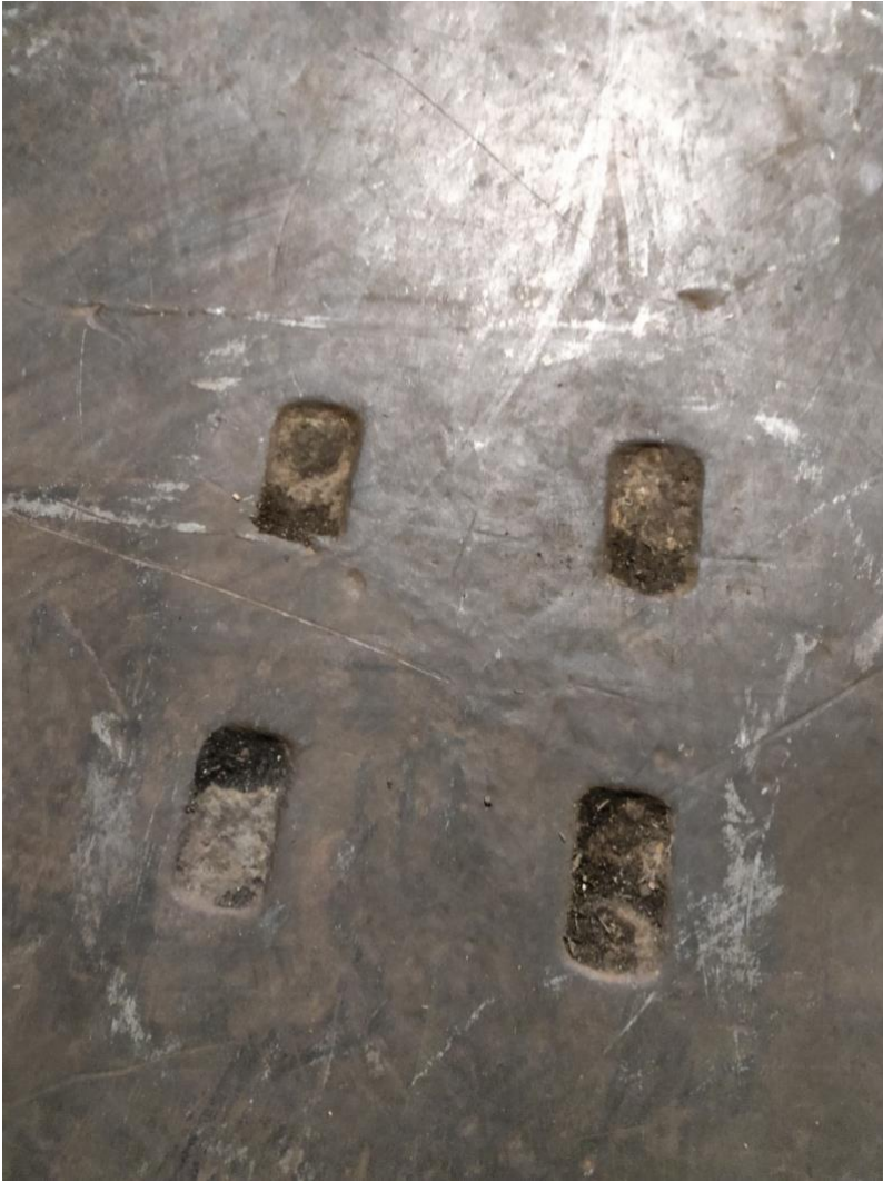
Figure 17 Tanktop container socket with damaged concrete and dirt (Matti Heinonen 2021)
