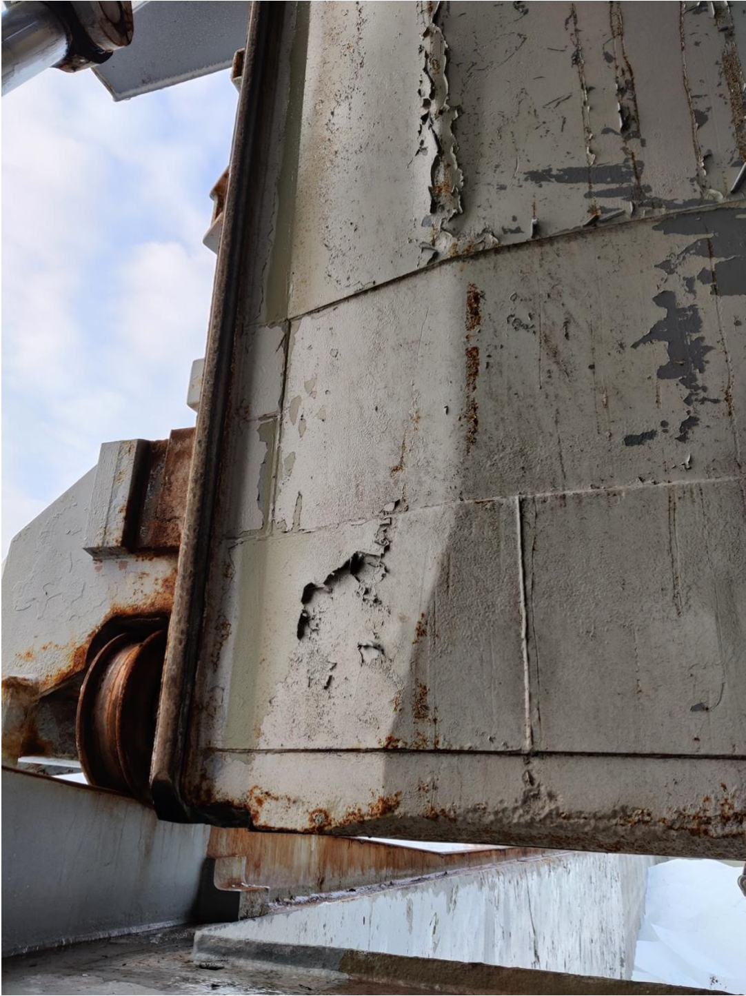
Figure 4 Loose paint on hatch cover (Matti Heinonen 2021)
