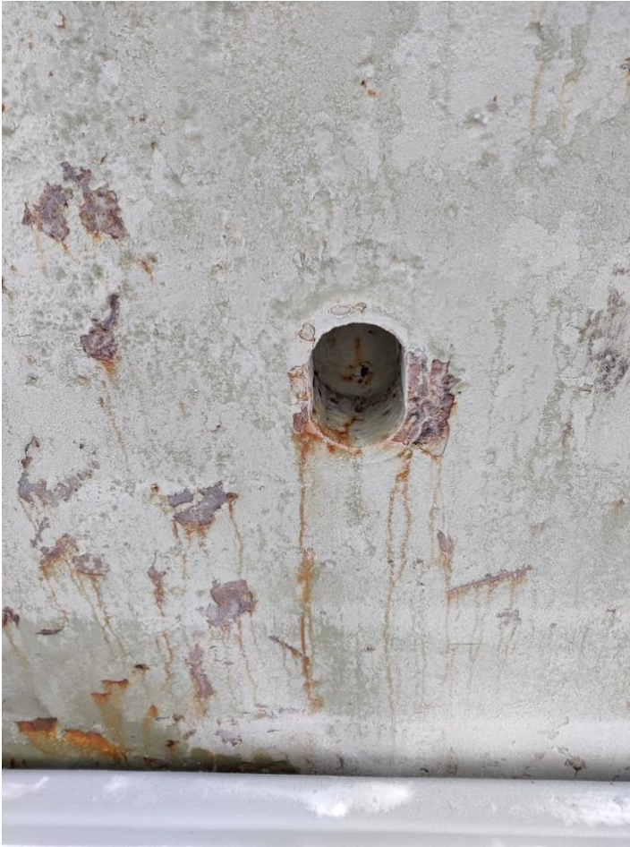
Figure 22 Bulkhead attachment socket. No cargo residues but some loose rust and paint. (Matti Heinonen 2021)
