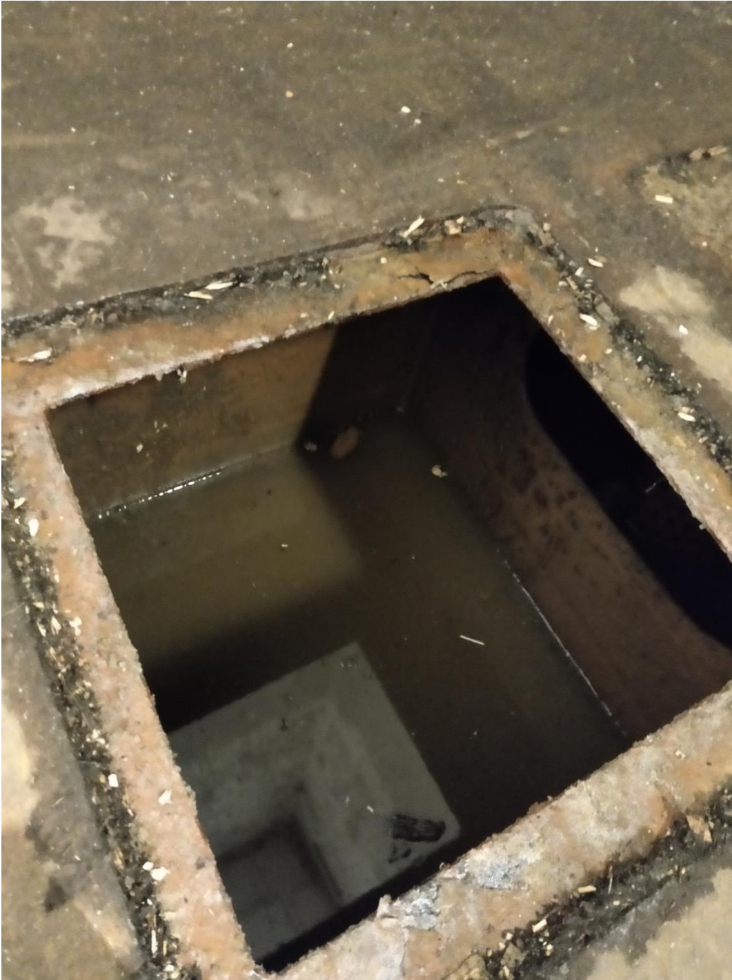
Figure 5 Bilge well full of water (Matti Heinonen 2021)
