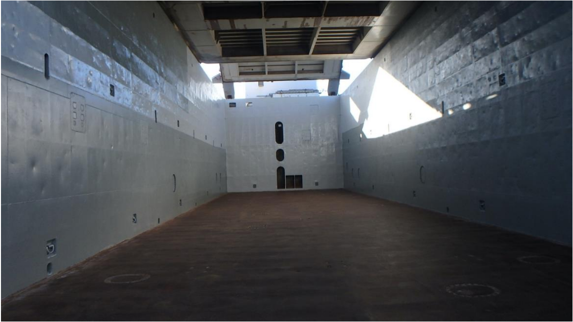
Figure 13 Optimal situation, freshly painted cargo hold during few days lay time at Ostend (Matti Heinonen 2020)
