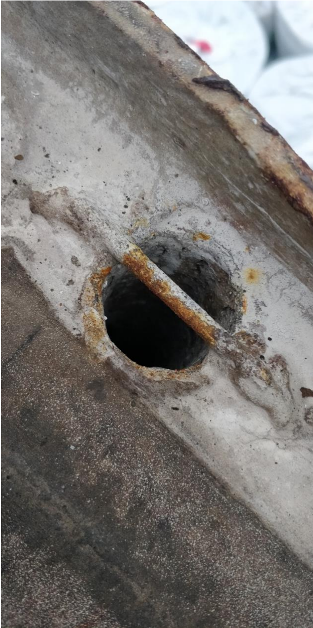
Figure 33 Draining pipe. (Matti Heinonen 2021)
