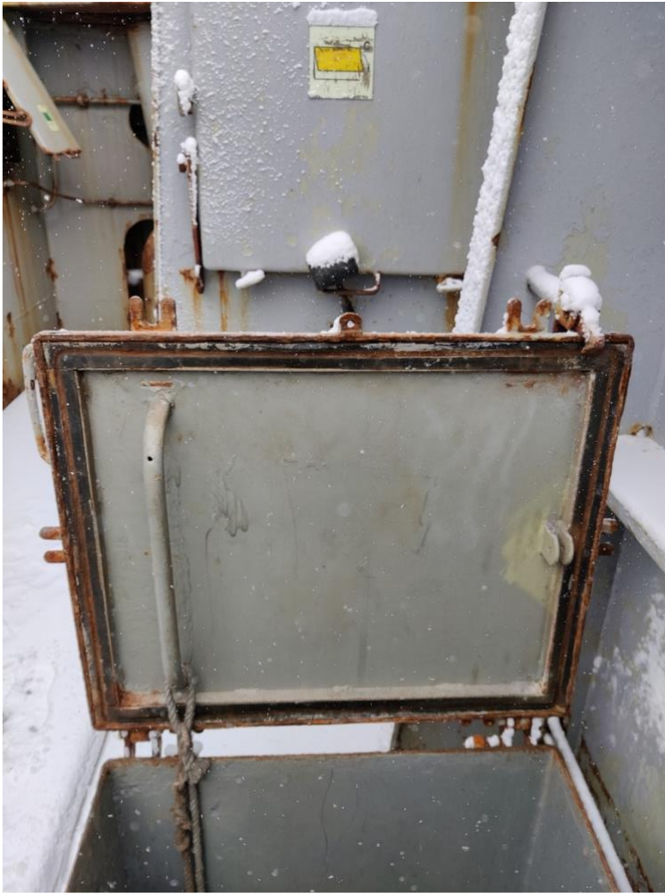
Figure 24 Forward cargo hold entrance. Sealing gasket to be checked. (Matti Heinonen 2021)
