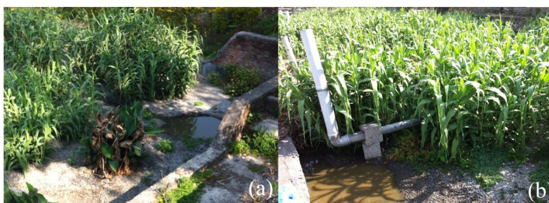
FIGURE 28. Ponding effect in Sunga constructed wetland WWTP; (a) HFB; and (b) VFB
