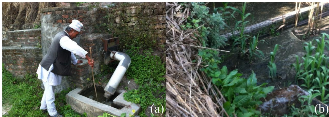
FIGURE 27. Sunga Constructed Wetland WWTP; (a) Caretaker cleaning the grit chamber; and (b) Over flow of wastewater from the top of HFB surface
