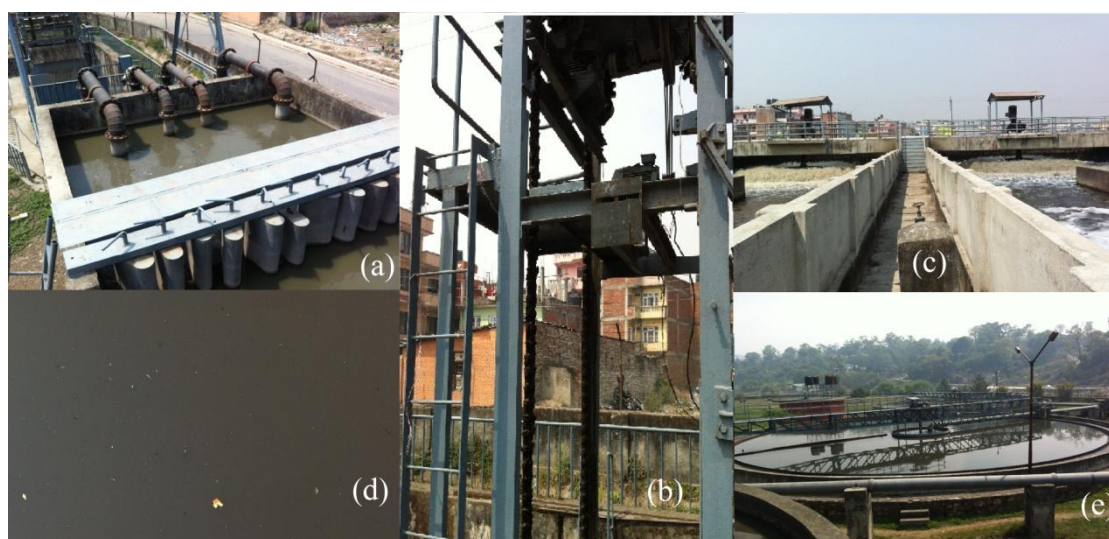
FIGURE 17. Different units of Guheshwori WWTP; (a) Usage of pump to pass the water through grit chamber; (b) Grab screen to remove large materials; (c) Blower aerators in action; (d) Feather like structures in settling tank; and (e) Settling tanks
