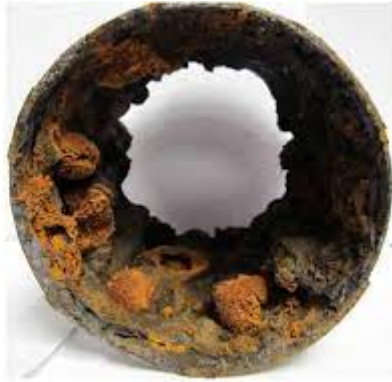
PICTURE 6. Microbiologically influenced corrosion (Tim O'Leary 2017)
