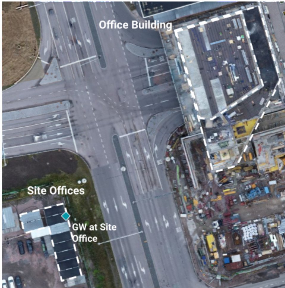
Figure 39. Top down view of the Tuultenristi construction site with outlines for the relevant buildings and site office.
