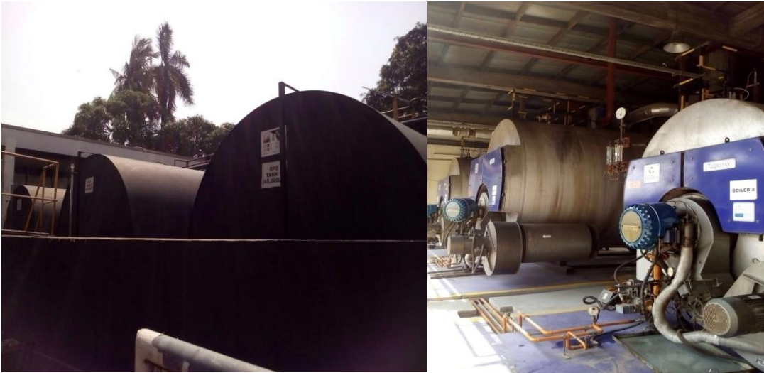
Figure 2. Boilers and fuel tanks
