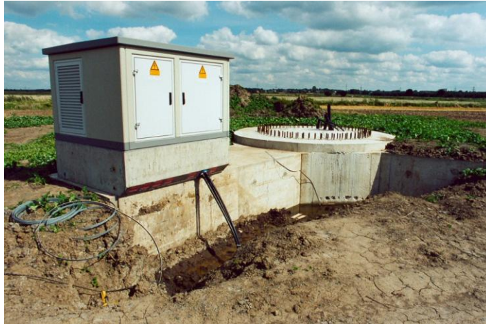
FIGURE 13: Foundation and transformer for a wind turbine. ©Bundesverband WindEnergie e.V. (World Wind Energy Association 2010)
