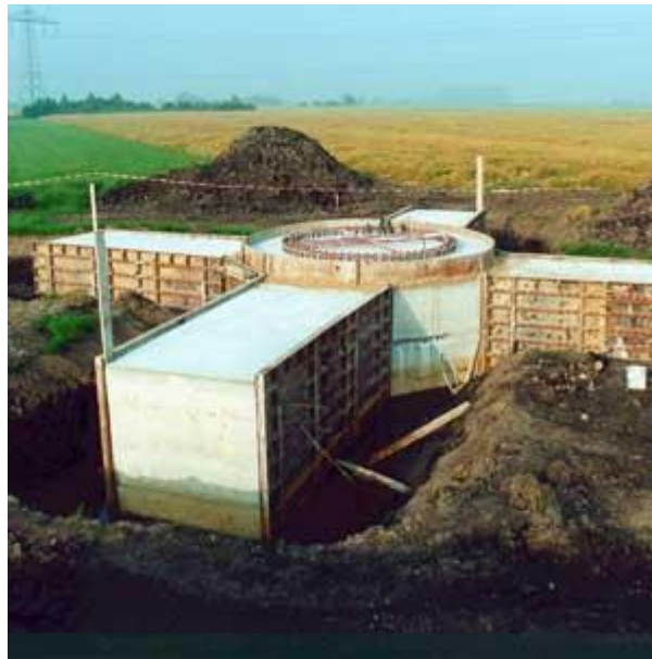
FIGURE 12: Foundation of the wind turbine is completed in Uetersen wind farm, Germany© Bundesverband WindEnergie e.V. (World Wind Energy Association 2010)
