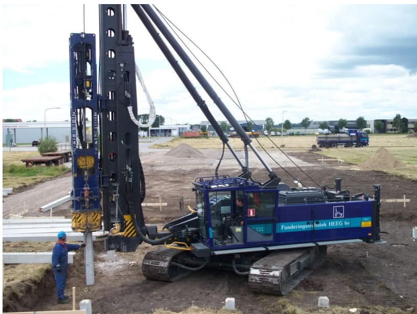
Picture 1 – A piling rig is driving a pile into the soil (Junttan Oy, product archive)
