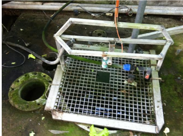
Picture 5 - Underground Water tanks
