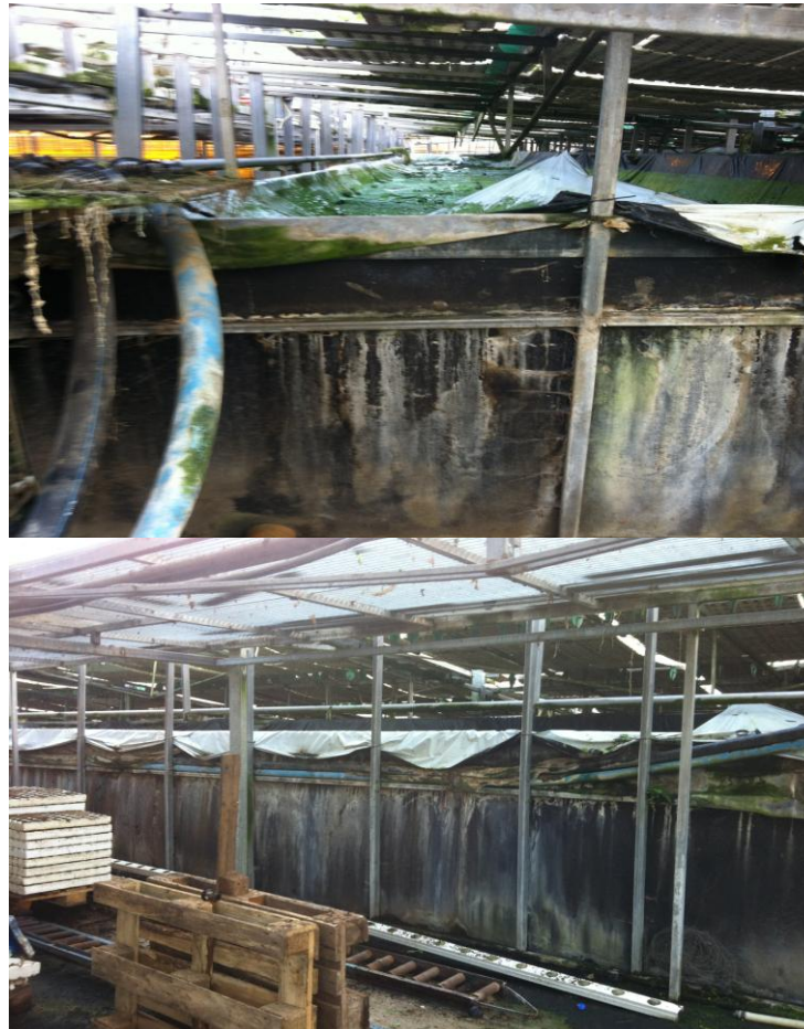
Picture 2- Sand filtration area
