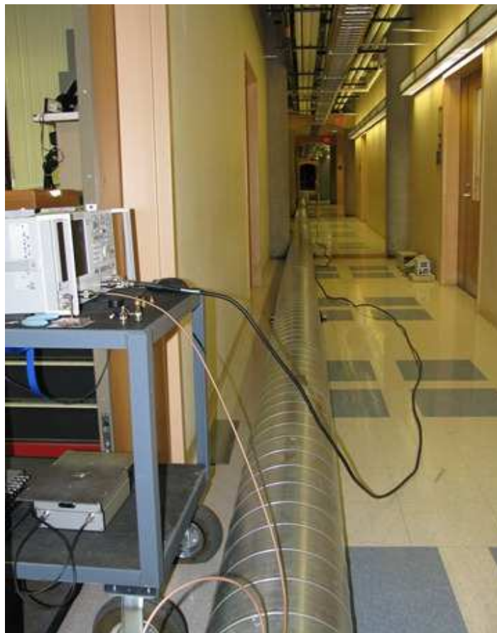
FIGURE 24. RFID Temperature smart sensor in a vent (Rfid.thingmagic 2012)
