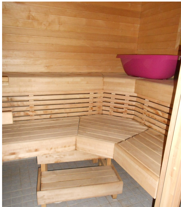
FIGURE 4: The Sauna in Villa Hiidenmäki: Handrails were missing.
