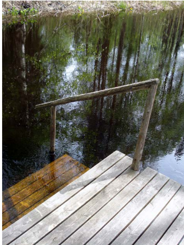
FIGURE 12: The railing of the platform was only on the right side
