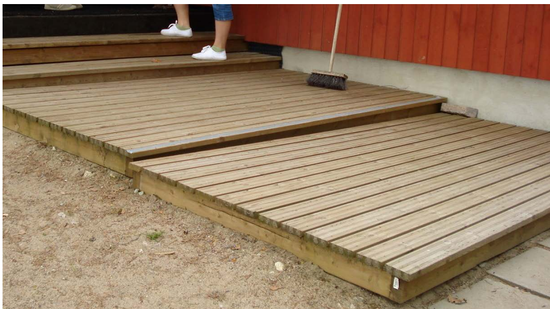
FIGURE 9. The staircase outside of Tähtitalvikki should be marked better to prevent accidents.
